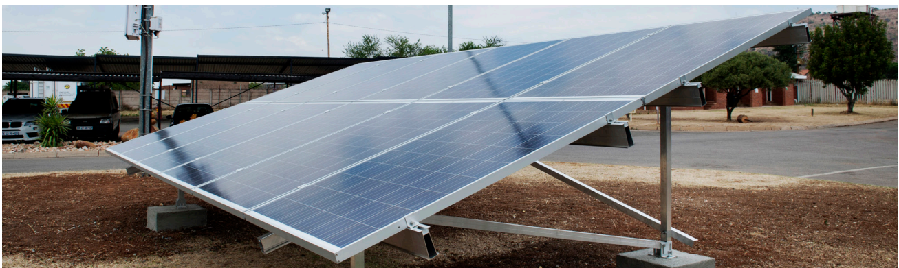
Ground mount PV module array; Photographer Manyatsa Monyamane, © GIZ
