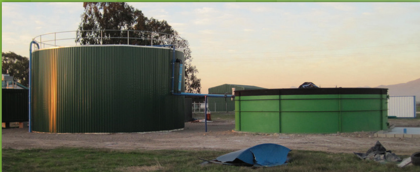
Figure 2: From left to right; storage tank, digester tank & CHP container
